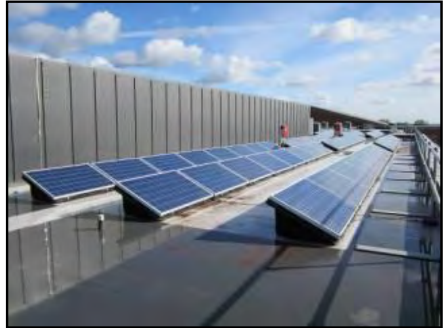
Solar PV installation at Queen Elizabeth School, Wimborne
