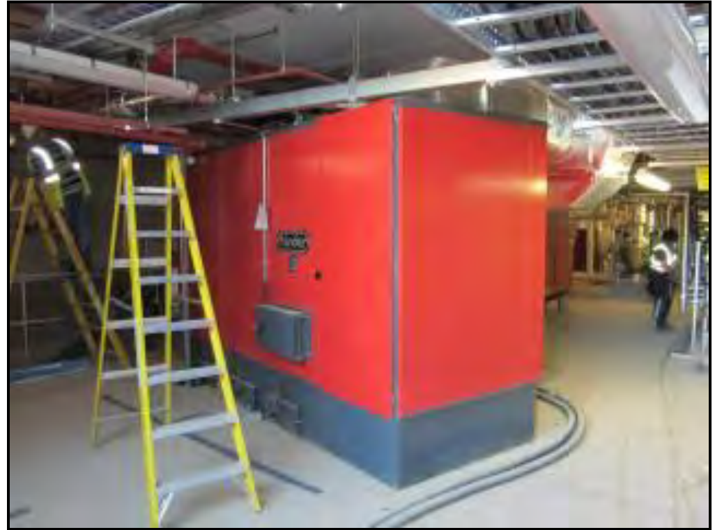
800kW woodchip boiler at Queen Elizabeth School, Wimborne
